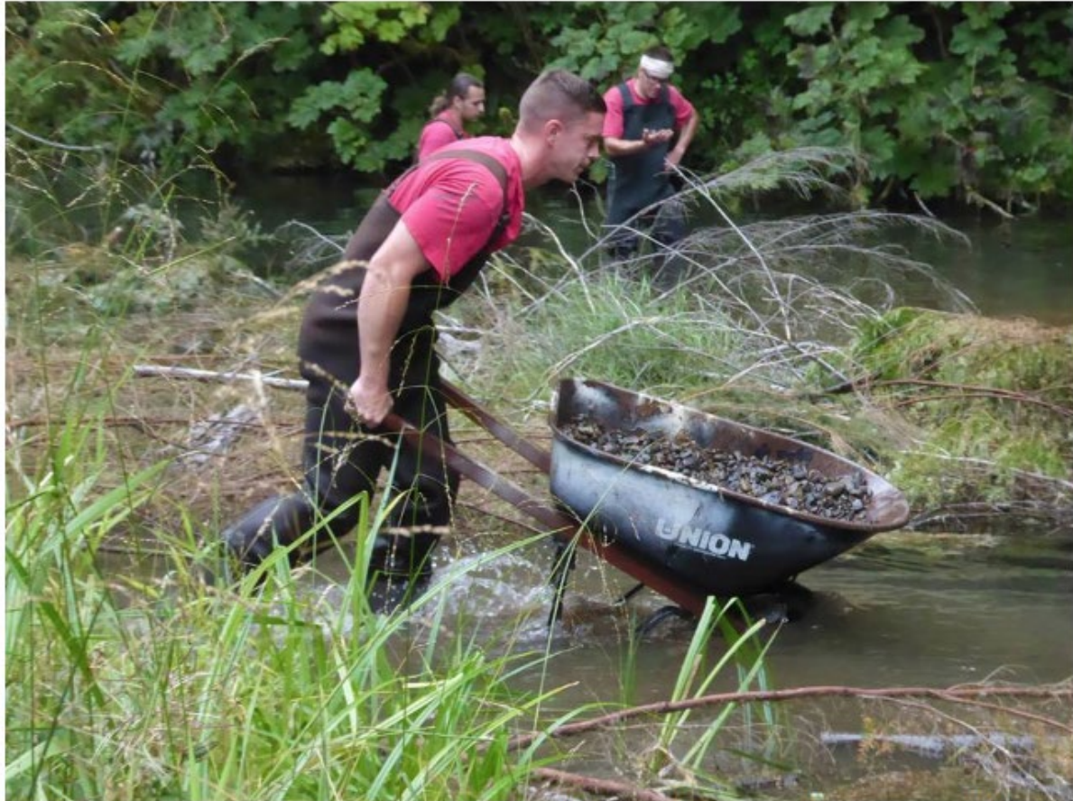
OCC inmate crew member places a wheelbarrow full of gravel in the creek. Photos David Hahn
